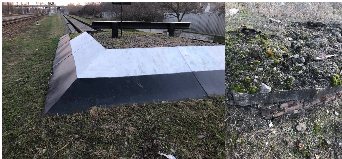
Blind area of the railway dead-end (site No. 6); Concrete slab on brickwork with construction outline, 2m from the railway track (site No. 2).
